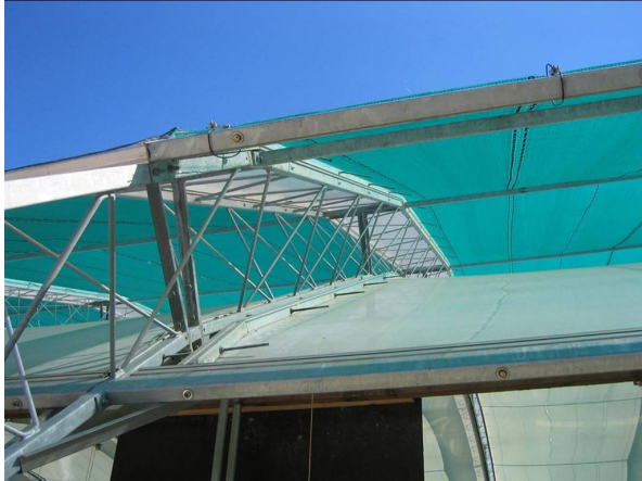
Figure 12 Detail of the roof: truss structure, upper and lower membrane and ventilation openings
